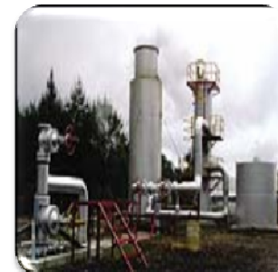
•Los Azufres, Geothermal Plant Michoacán
